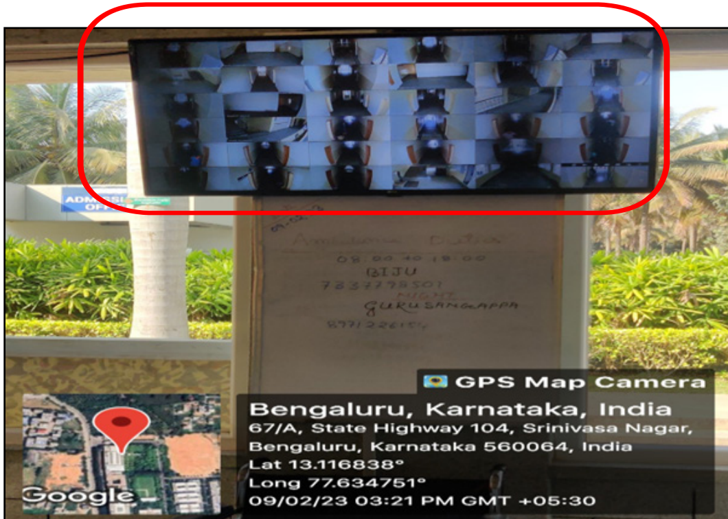
CCTV surveillance at Main Gate
