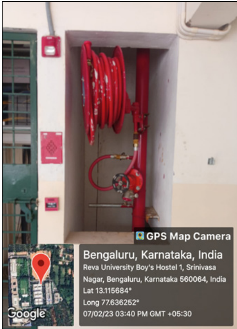
Fire extinguisher system
