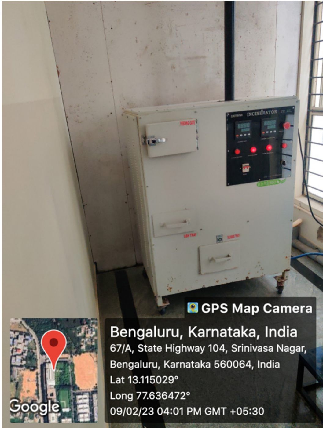
Incinerator machine, Girls hostel REVA University
