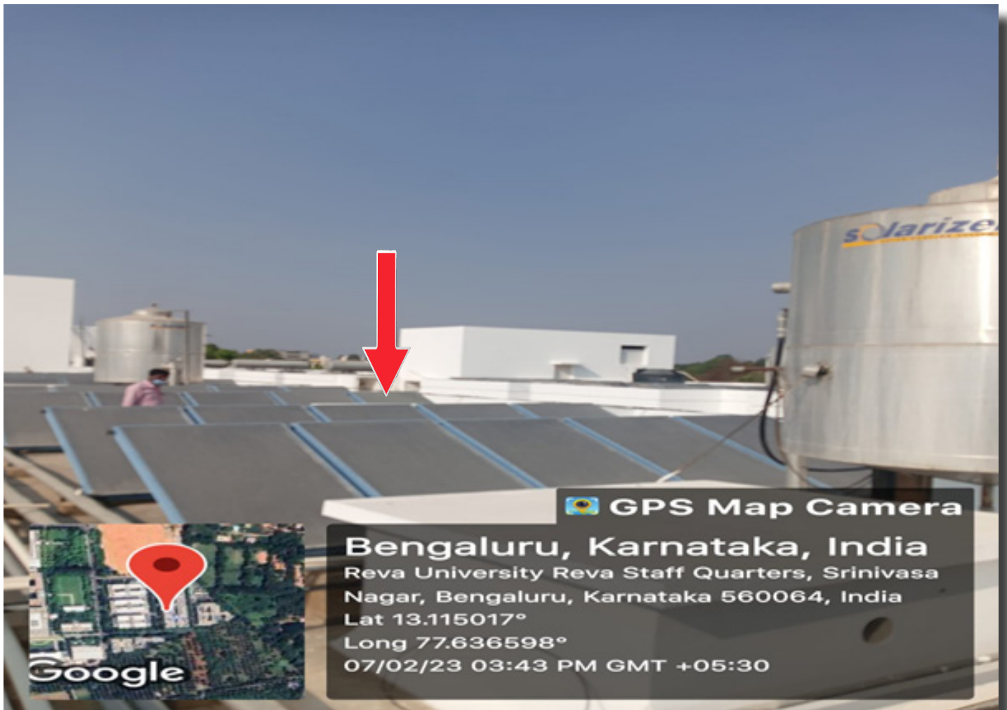
Solar Energy System Block: Administration
