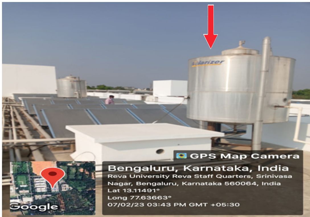
Solar Energy System Block: Administration
