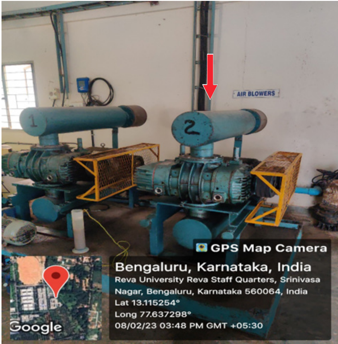
Air Blowers in filtration unit Block: Sewage Treatment Plant, REVA University
