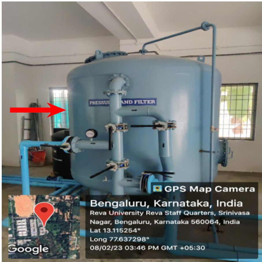
Water Filtering Units Block: Sewage Treatment Plant, REVA University
