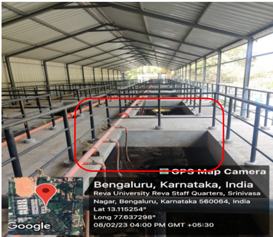
Stagnation of wastewater within the plant Block: Sewage Treatment Plant, REVA University
