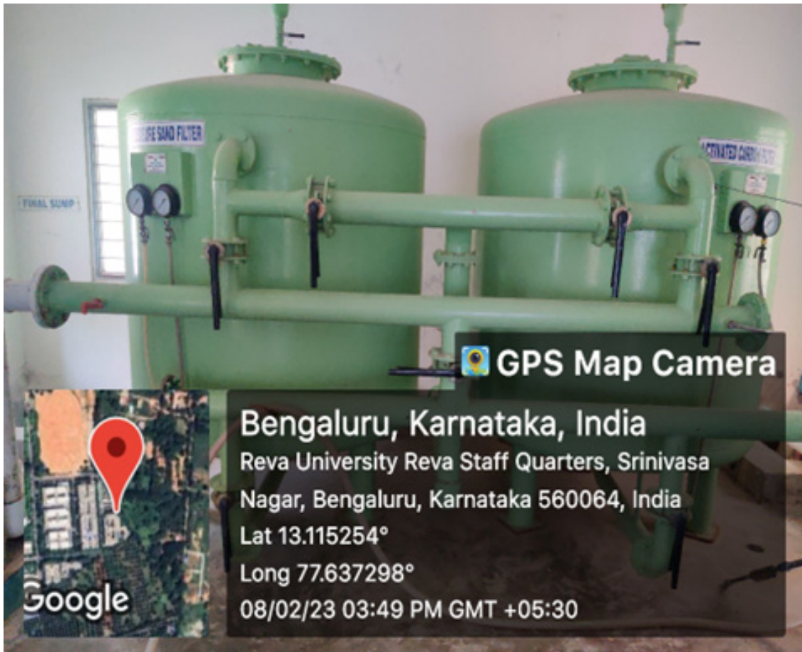
Final sump with activated carbon and sand filtes Block: Sewage Treatment Plant, REVA University
