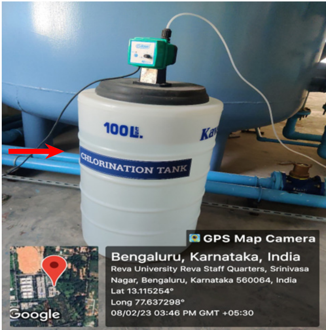
Chorination Tank for water filtration Block: Sewage Treatment Plant, REVA University
