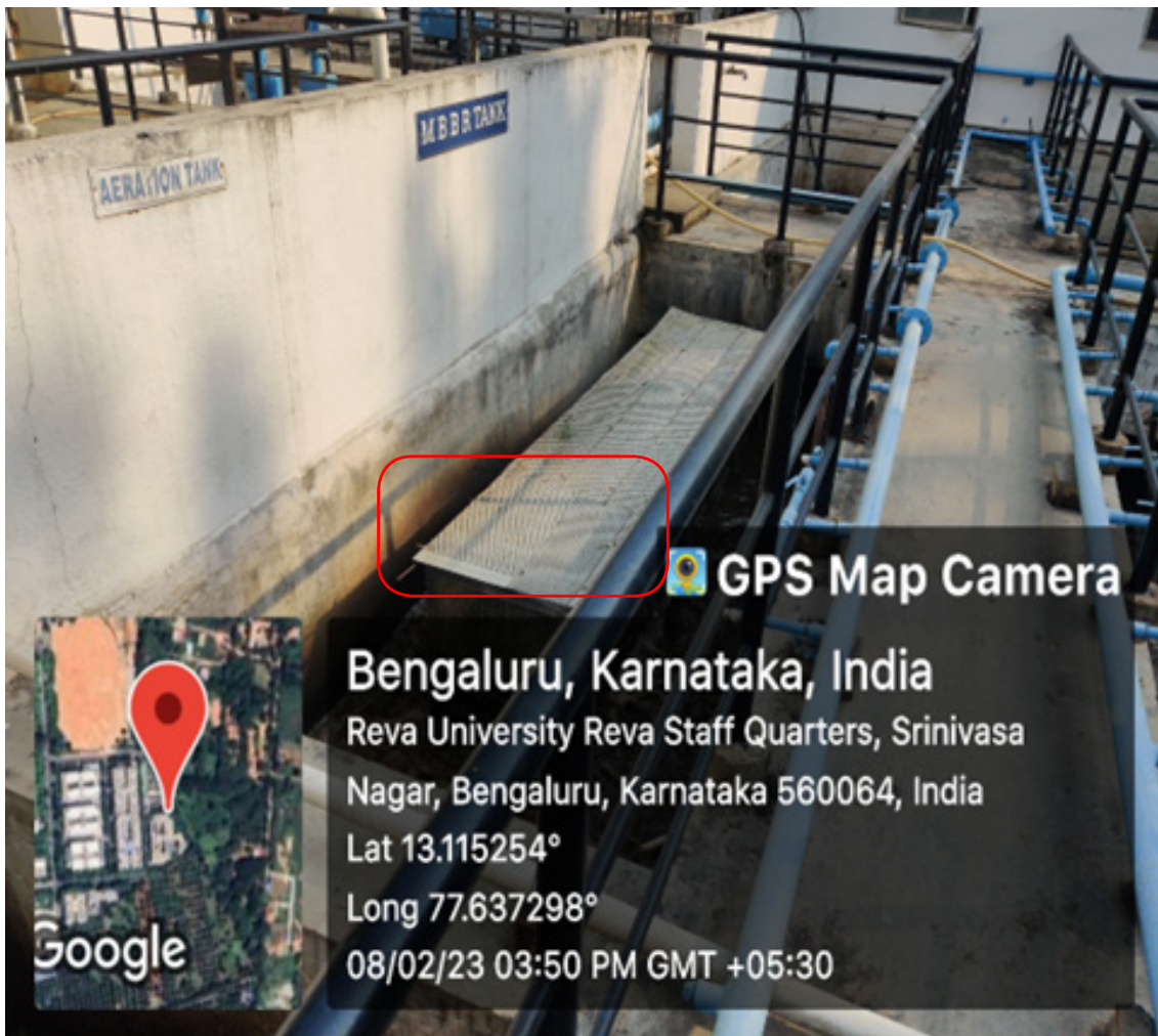
Water sump Block: Sewage Treatment Plant, REVA University
