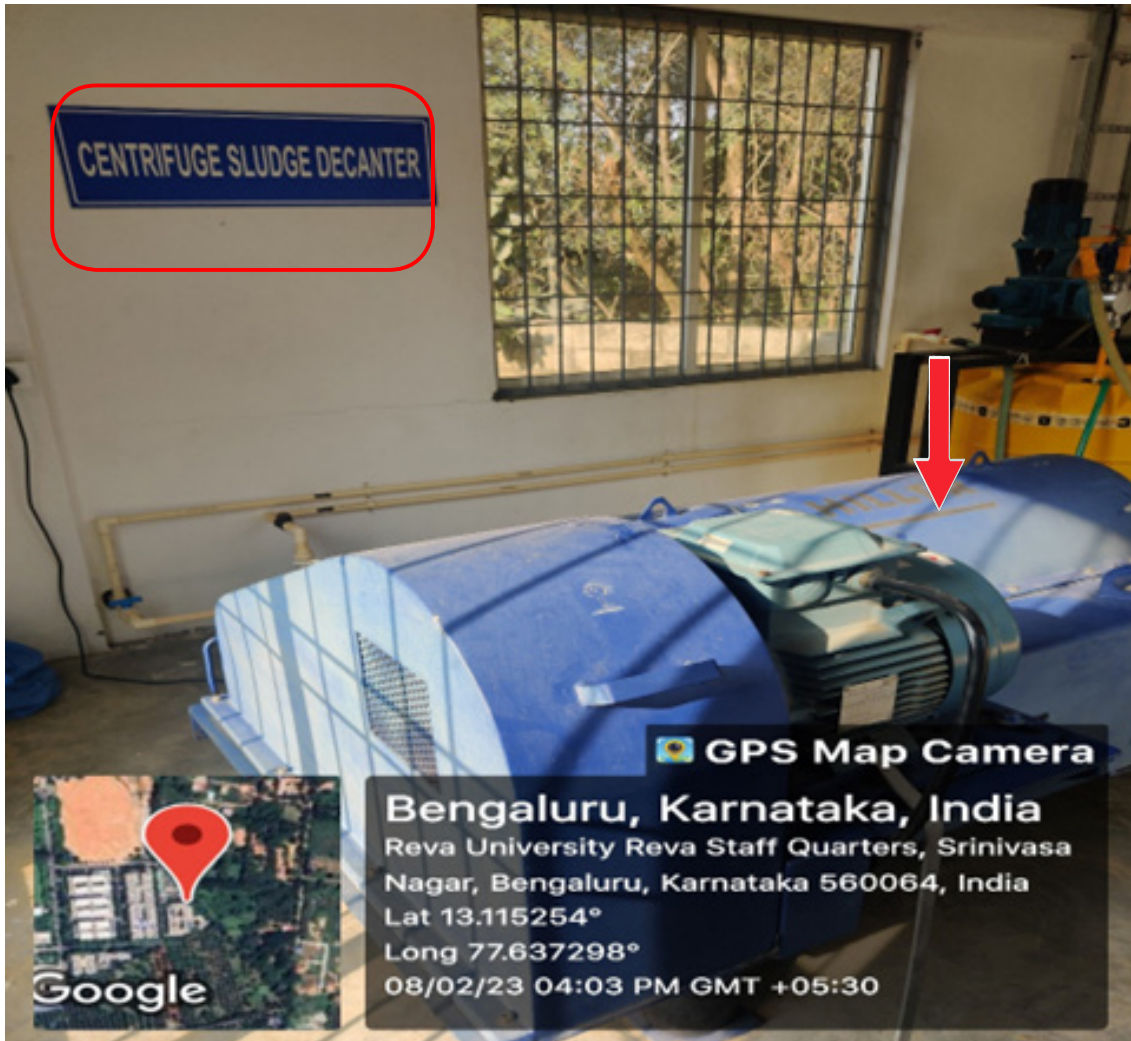
Sludge Decander to separate liquid waste and solid waste Block: Sewage Treatment Plant, REVA University
