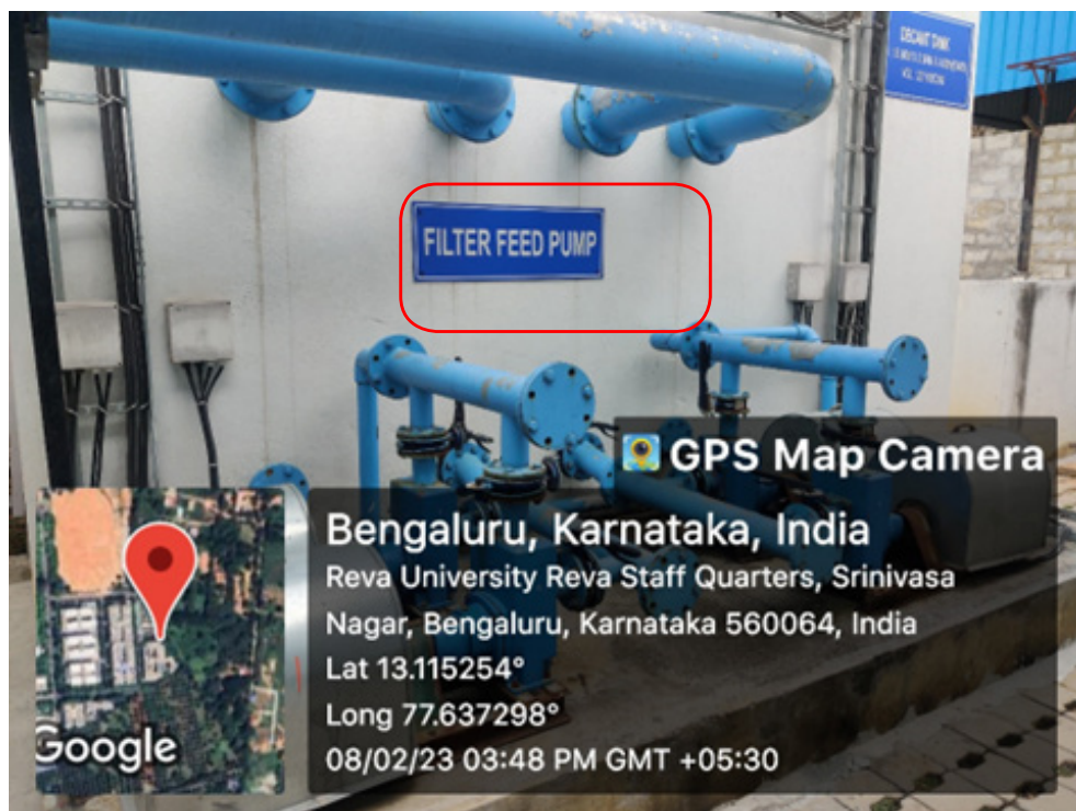
Filtered feed unit to pump waste water Block: Sewage Treatment Plant, REVA University
