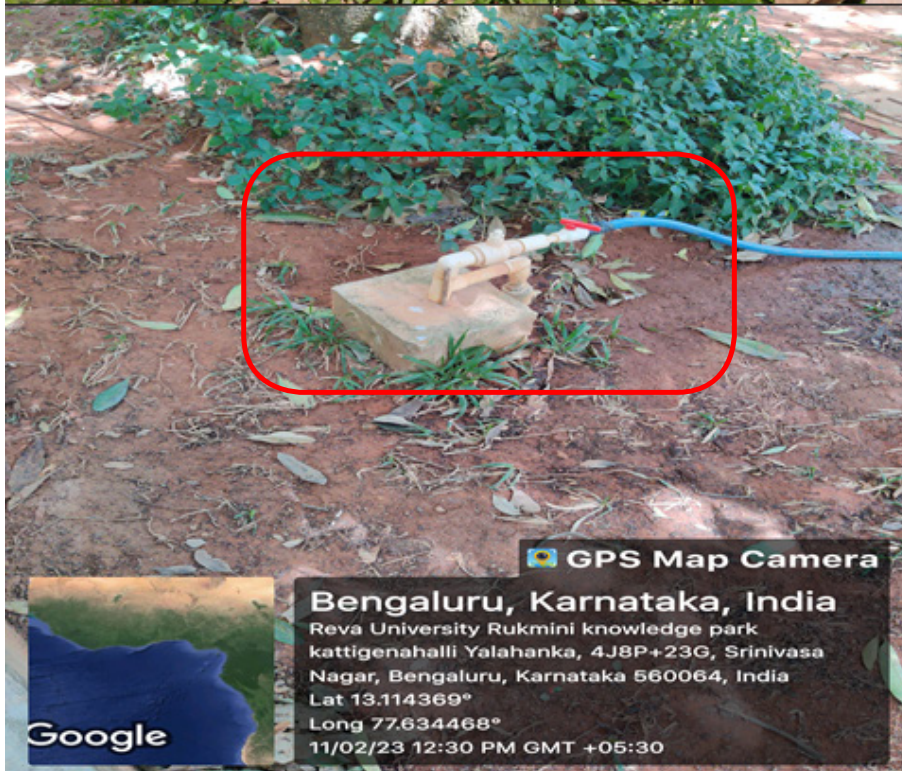
Borewell recharge system and distribution points Block- Science and Swami Vivekananda, REVA University
