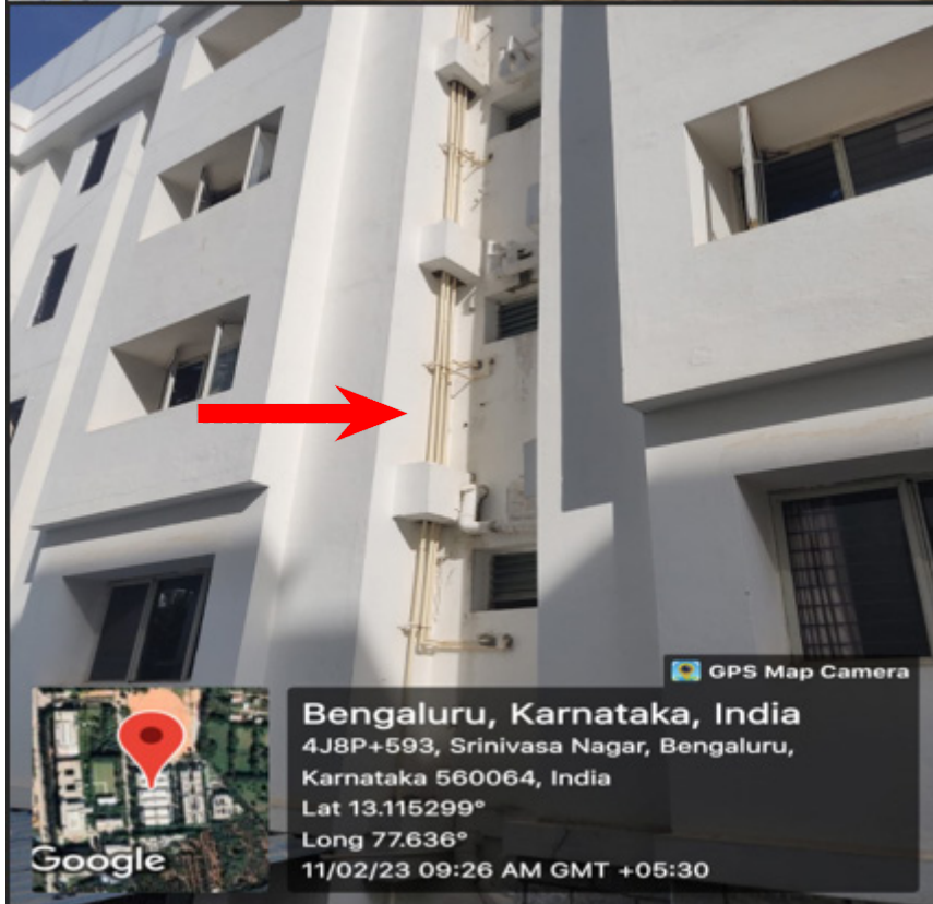
Water distribution Block- REVA Students Hostel
