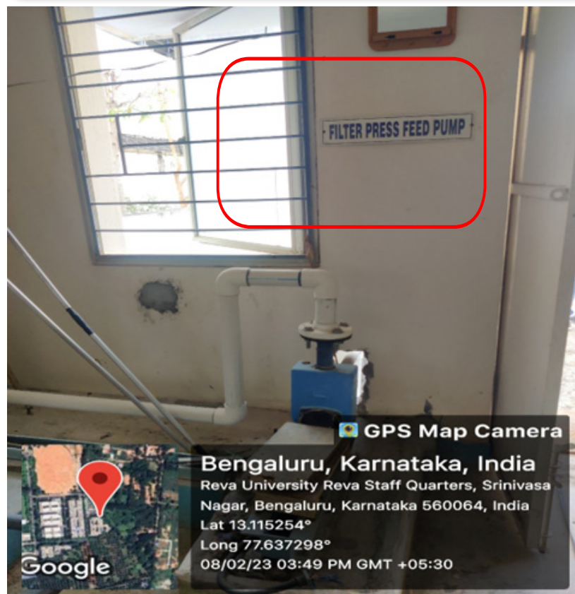
Wastewater stagnation block and filter feed pump Location: Sewage Treatment Plant, REVA University
