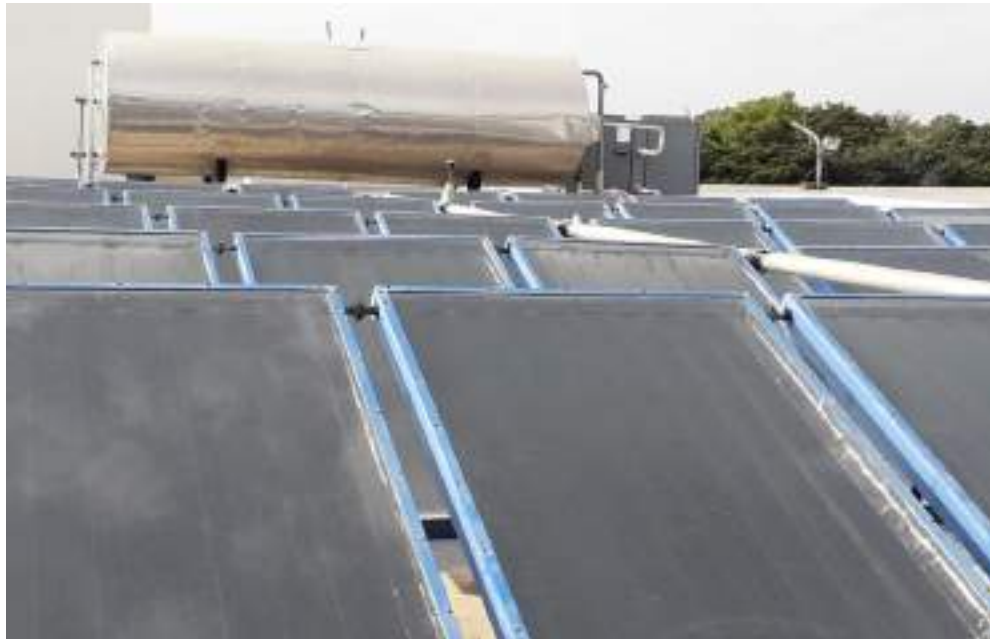
Figure 46: View of Solar water heater system installed at REVA Campus.
