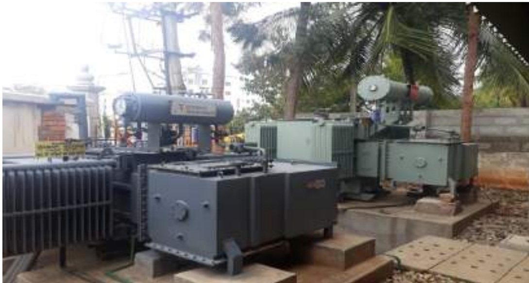
Figure 31: View of sub-station & transformer yard.
