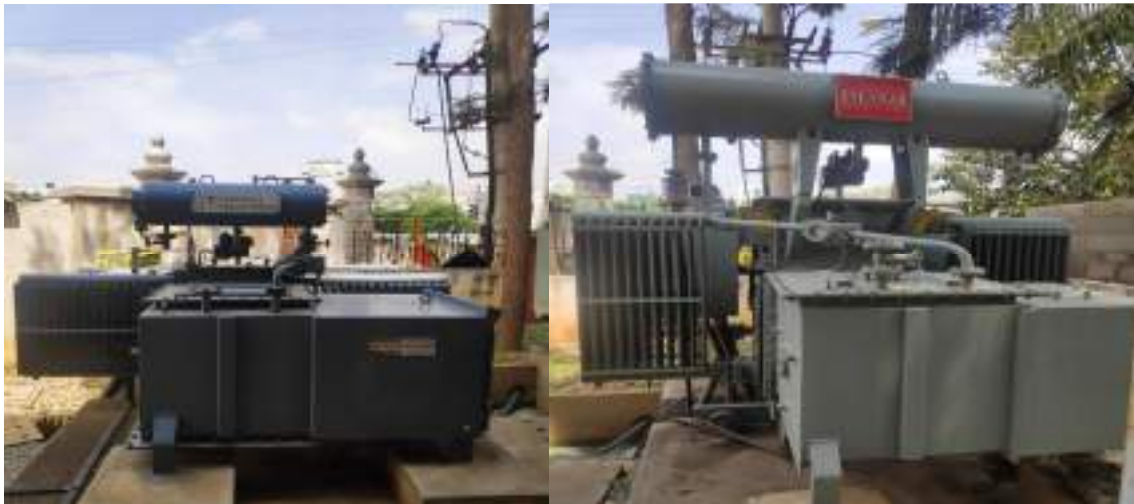
Figure 29: View of main Tr.1 (500 kVA) Figure 30: View of main Tr. 2 (1000 kVA)
