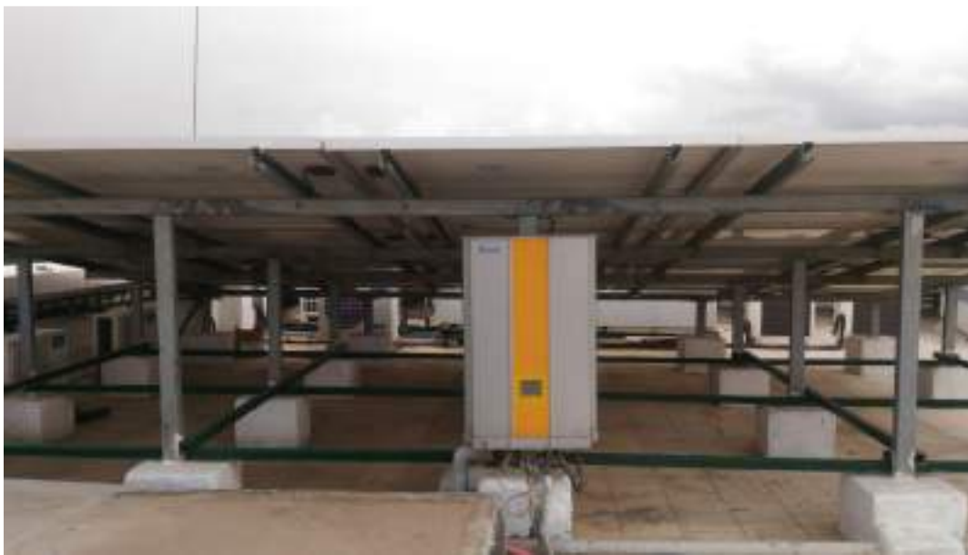
Figure 35: View of inverters of 55 kW Solar PV power plant at Admin Block
