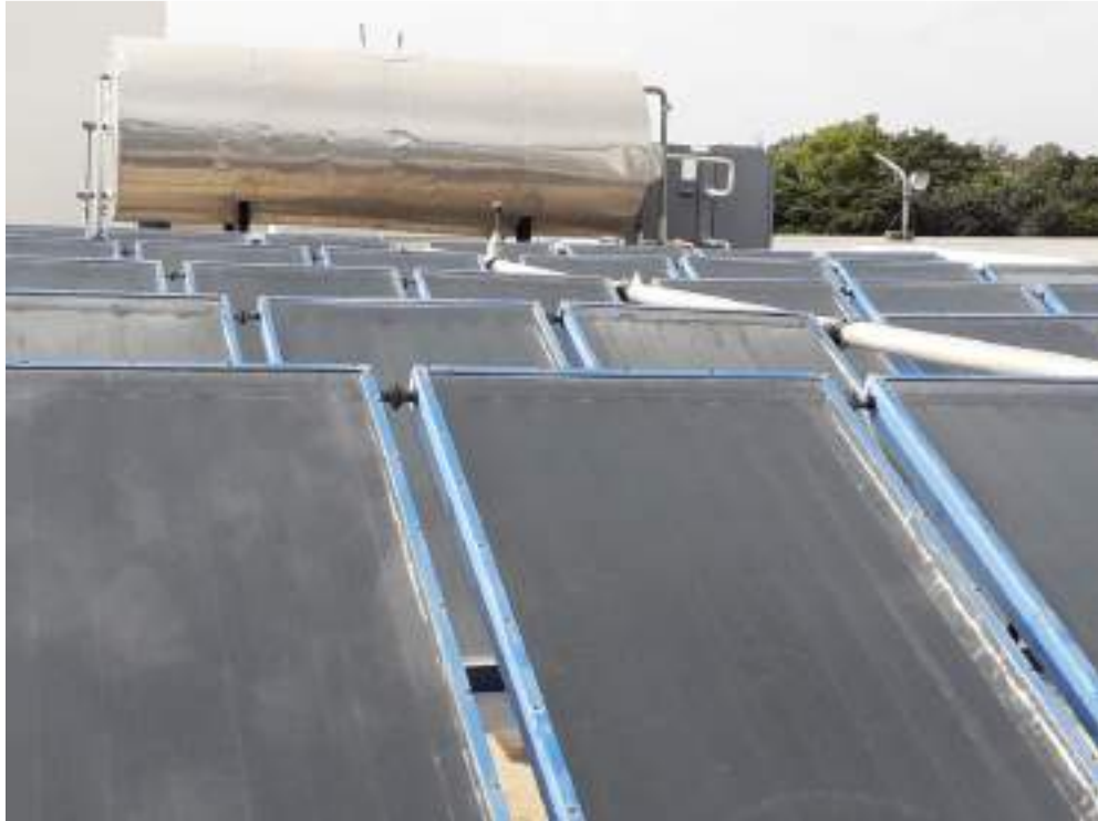
Figure 47: View of Solar hot water system.
